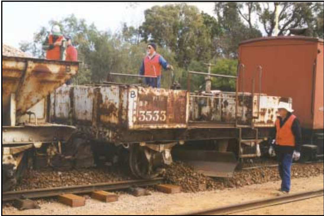
First drop ballasting along the platform road at Port Augusta Station using ex S.A.R. Port Lincoln Division plough BP3533 and 12 four wheel hoppers.
