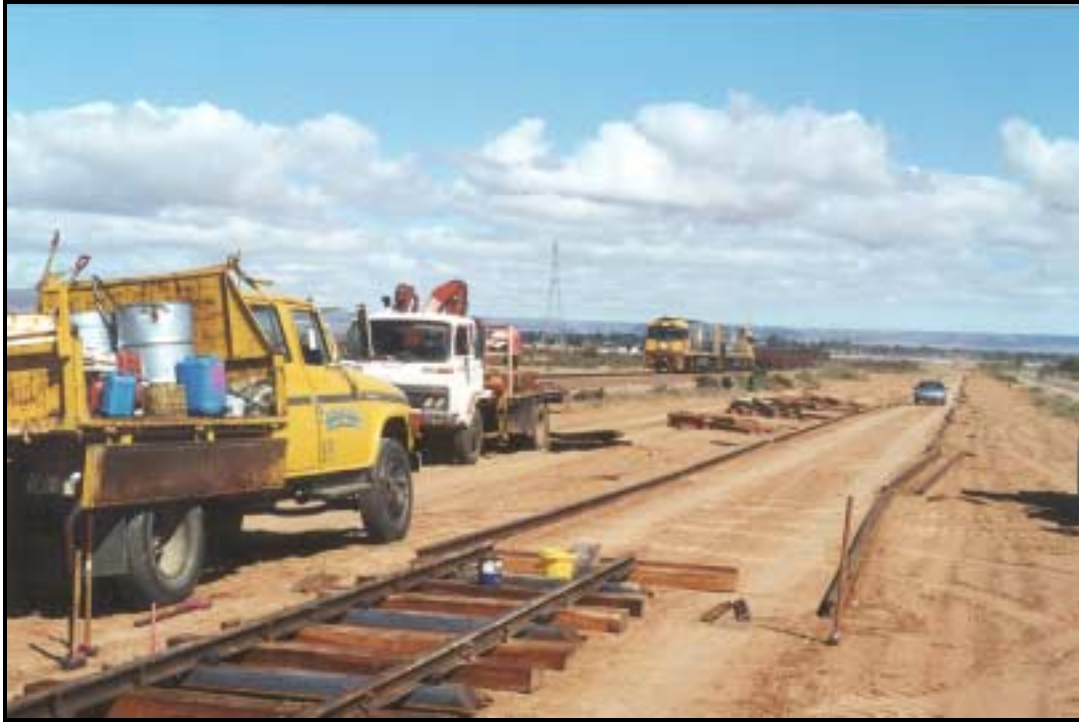
Early track construction between Harris Street and Footner Road. Note the 1 in 3 steel sleepers.
