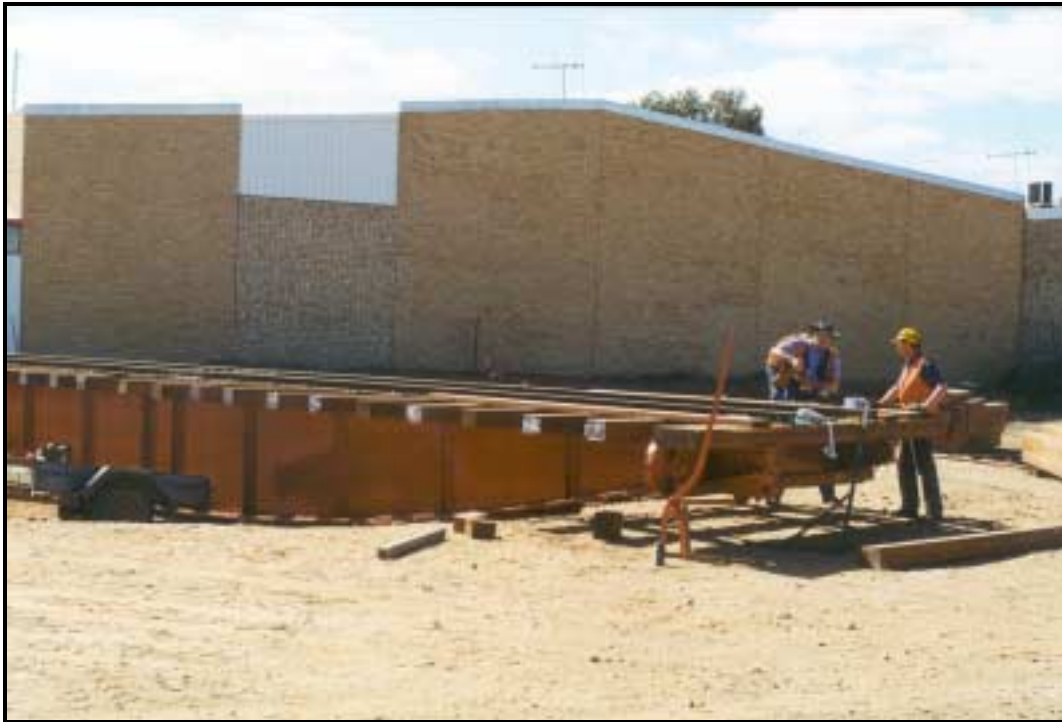
Volunteers from the Puffing Billy Railway, Victoria dressing timbers on the newly positioned turntable, opposite the old CR Stores Building on Railway Parade, Port Augusta
