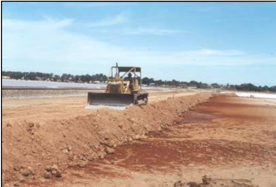
Trimming the top of the widened embankment across Lake Knockout. A local contractors vintage Cat D5 dozer was more than adequate.
